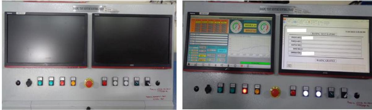
Figure 22. Pressure Test System Control Board
