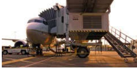
Figure. 1. Jetway-mounted HVAC system: PCA. (Airport Systems, 2016).
