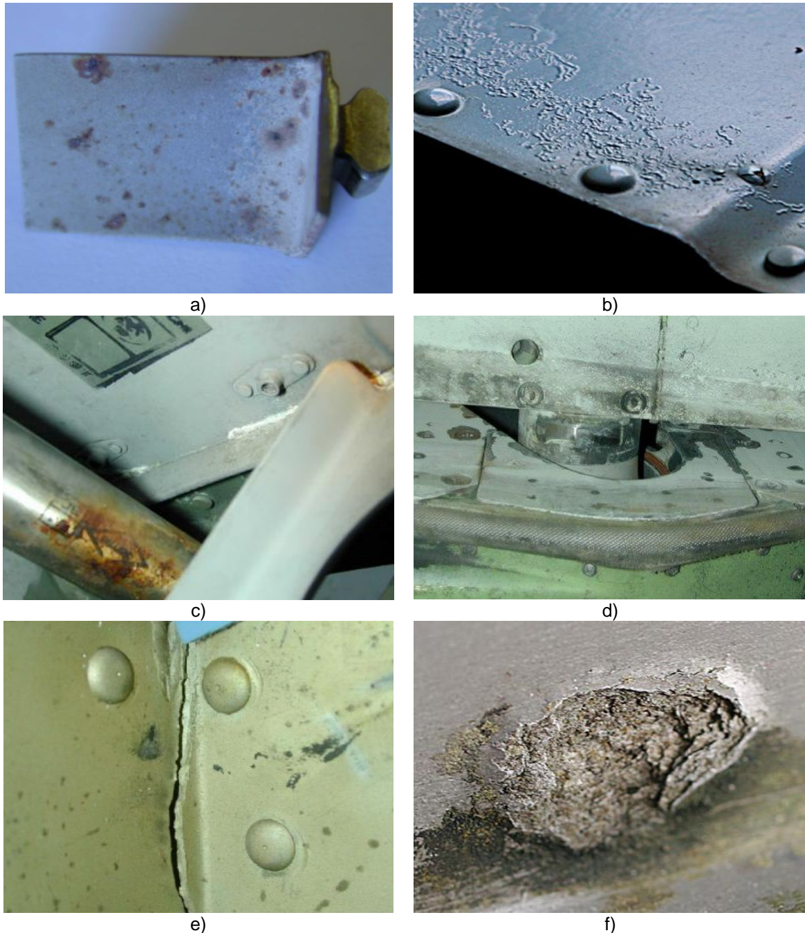
Figure 1: Various Types of Corrosion, a) Pitting Corrosion [Colavita, 2013], b) Surface Corrosion, c) Dissimilar Corrosion [Colavita, 2013], d) Fretting Corrosion [NACE, 2013] e) Stress Corrosion, f) Inter-granular Corrosion.
